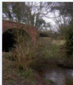
As the Oxford Canal passes Brinklow it had to cross a valley, so James Brindley designed an aqueduct to achieve this. There were twelve arches, each with a 22ft span. It is only possible to see one complete arch now, the one over the Smite Brook. Next to it is the top of a second arch.
